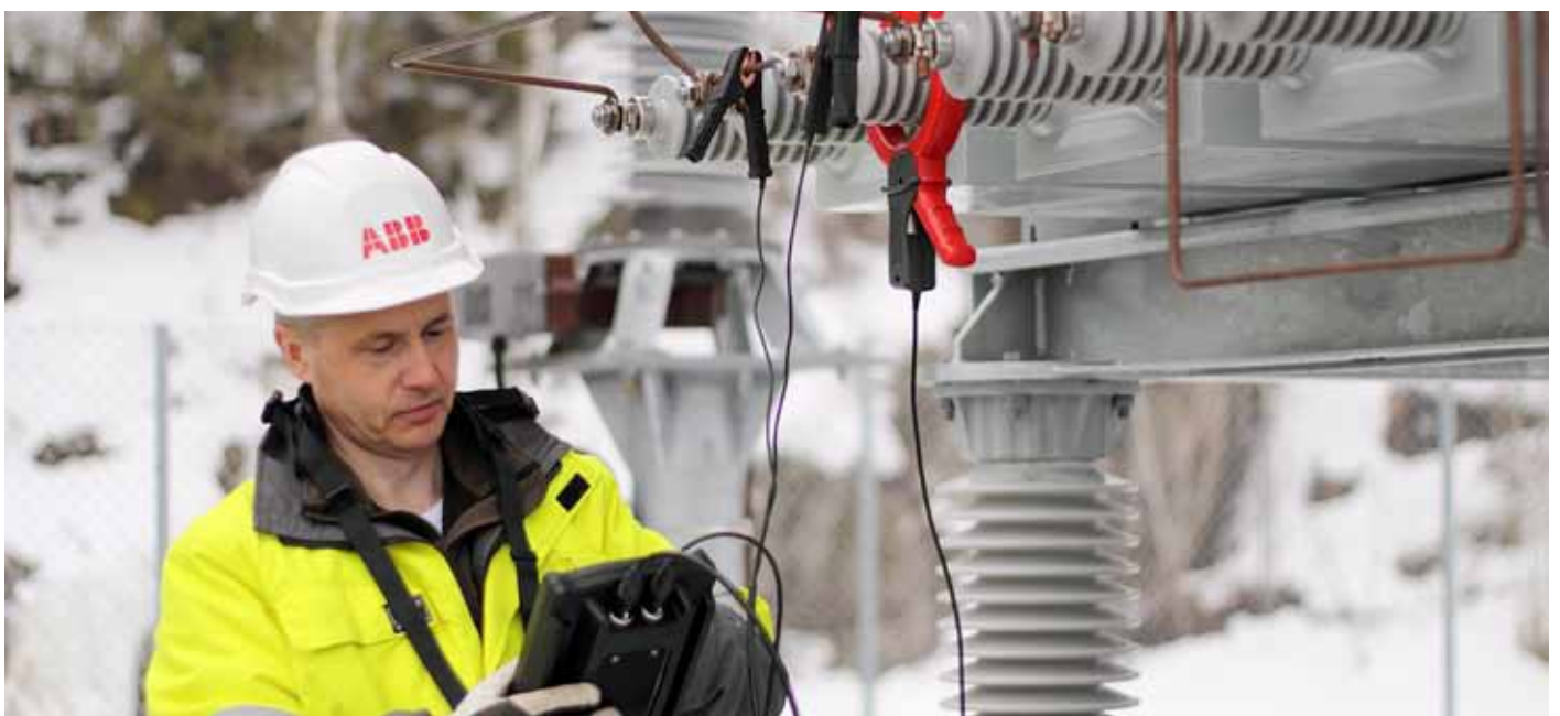
Measuring of capacitance in capacitor bank, Norway
