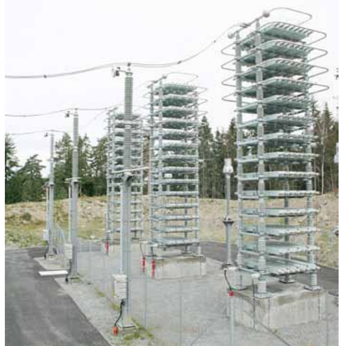
420 kV capacitor bank installation in Norway.
